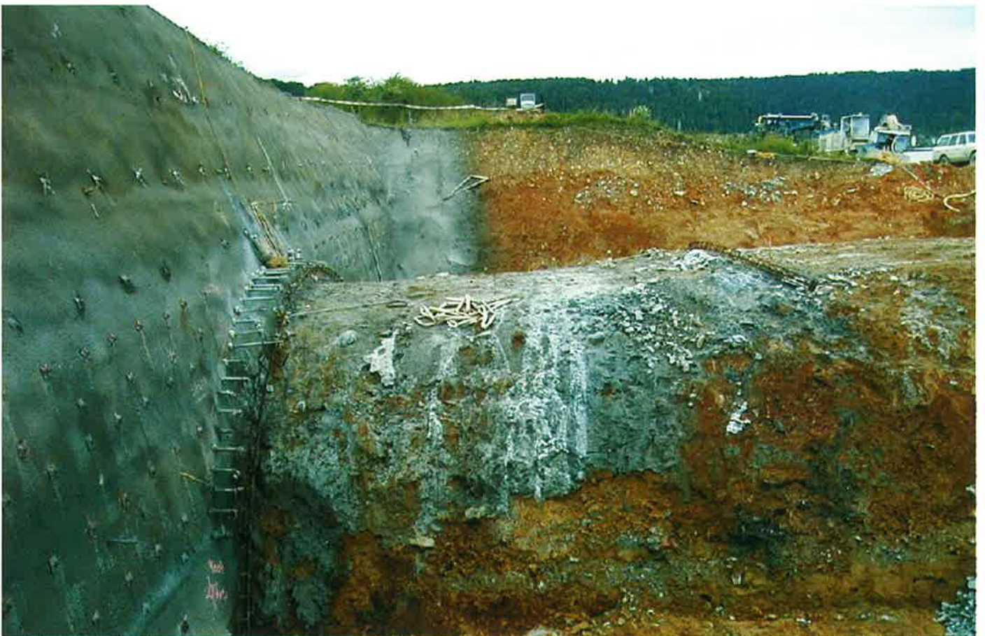
Obr. 11 Tunel Schellenberg – rozhraní želva – ražený tunel Fig. 11 The Schellenberg tunnel – the arch and mined tunnel contact area
