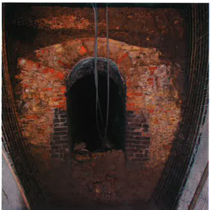
Obr. 3 Detail polohy Tereziánské štoly v průřezu tunelu Fig. 3 Detail of the position of the Theresian gallery within the tunnel cross section
