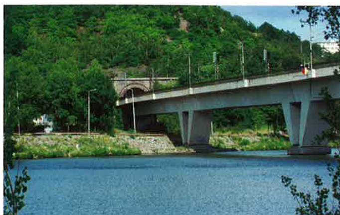
Obr. 5 Most a tunel pod Bílou skálou (1970) Fig. 5 Bílá skála railway bridge and tunnel
