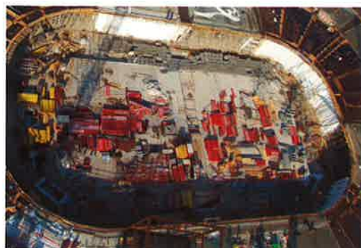
Realizace hokejové haly Sazka v Praze Construction of the Sazka Ice-hockey Arena in Prague
