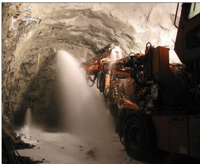
Obr. 2 Tlaková podzemní voda v tunelu Ólafsfjörður Fig. 2 Pressurised underground water in the Ólafsfjörður tunnel
