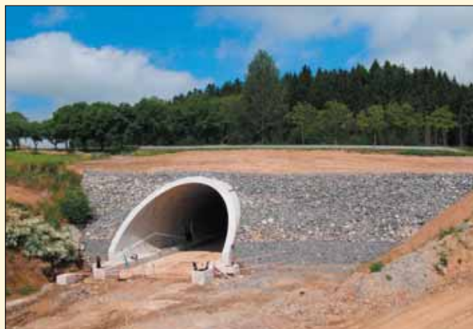
Obr. 3 Tunel Deboreč, pohled na vjezdový portál Fig. 3 Deboreč tunnel, view of entrance portal
