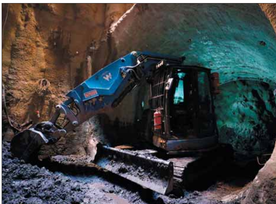
Obr. 9 Ražba štoly strojem BLUE BADGER Fig. 9 Gallery excavation using BLUE BADGER excavator
