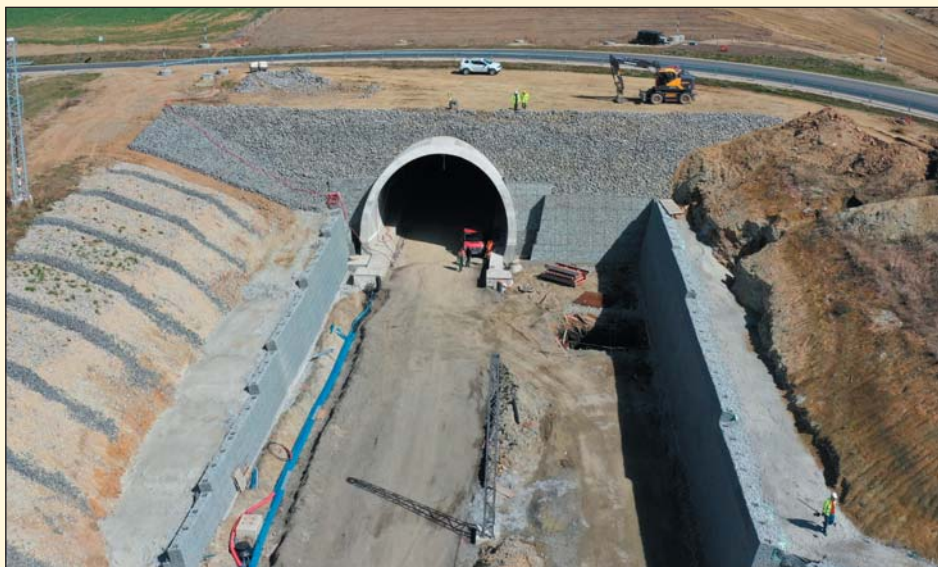
Obr. 2 Gabionové zdi na vjezdovém portále Fig. 2 Gabion walls at the entrance portal
