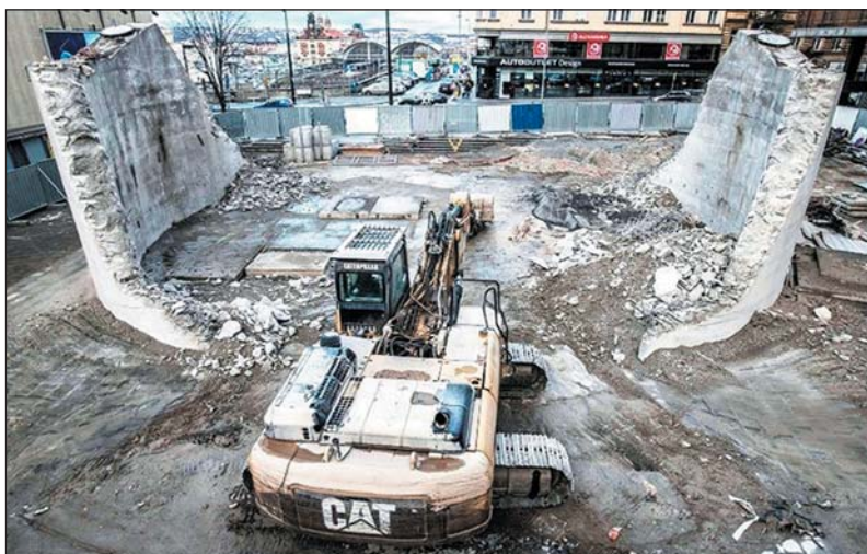
Obr. 6 Demolice vstupní budovy C Transgasu Fig. 6 Demolition of Transgas entrance building C
