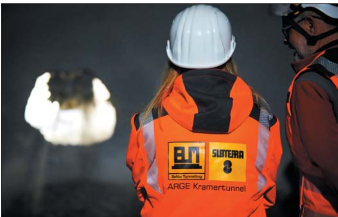
Obr. 5 Proražení tunelu tunelovací frézou pod dohledem patronky tunelu Fig. 5 Tunnel breaking through using a cutter boom under the supervision by the patron saint of the tunnel
