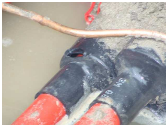
Obr. 5 Prasknutá tesniaca hadica, tzv. zmršťovacia Fig. 5 Split shrink sealing pipe
