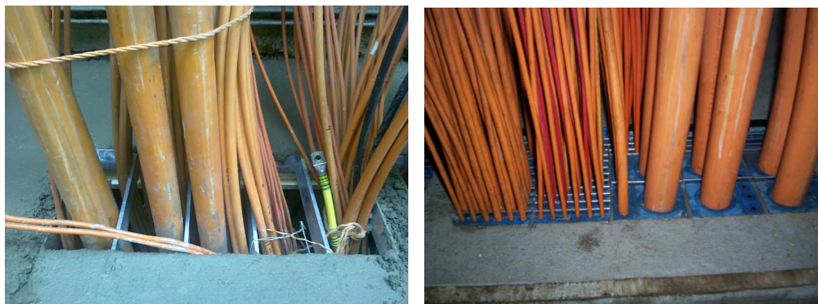
Obr. 3 Zaliatie tesniaceho rámu do betónu a utesnenie káblov modulmi Fig. 3 Concreting of the sealing frame and sealing - off cable modules
