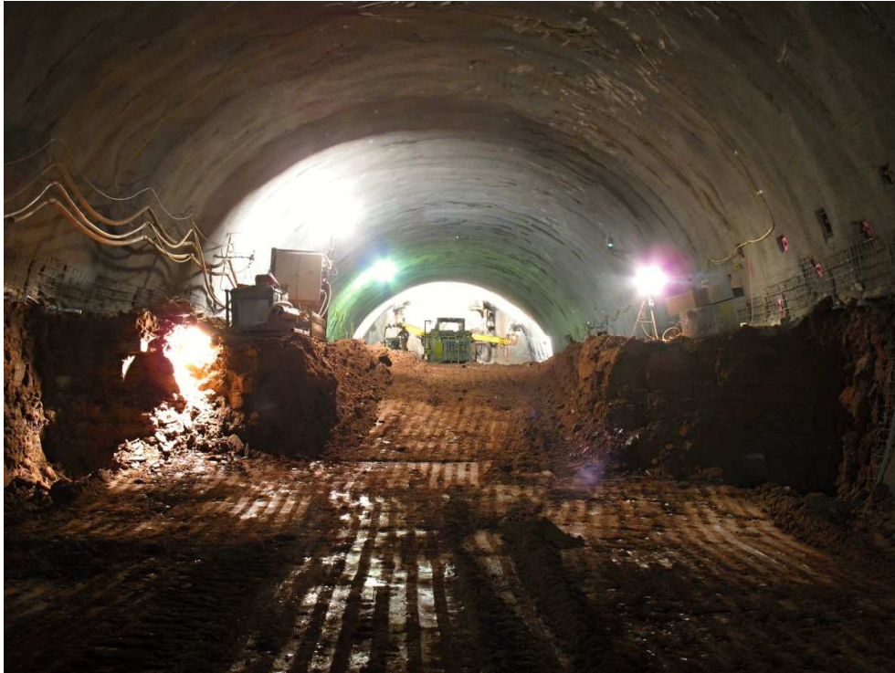
Obr. 4 Rampa v delenej lavici Fig. 4 Drive - up ramp in the vertically split bench
