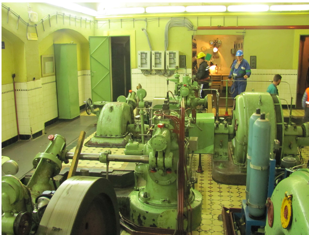
Obr. 1 Podzemná vodná elektráreň v hĺbke 245 m pod povrchom Fig. 1 Underground hydropower plant at a depth of 245 meters below the surface
