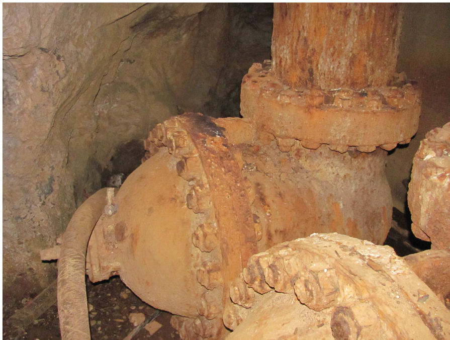
Obr. 4 Uzatváracie ventily na dne jamy č. IV Fig. 4 Shut-off valves on the bottom of the pit No. IV
