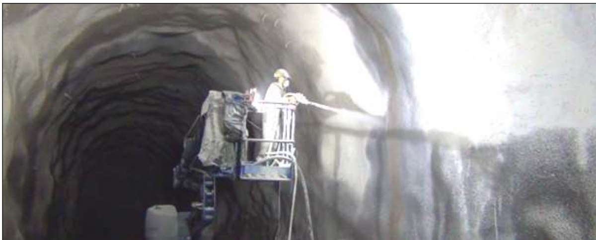
Obr. 2 Ostenie typu SSL v tuneli Skillingsmyr. Fig. 2 SSL Linings in Skillingsmyr tunel.
